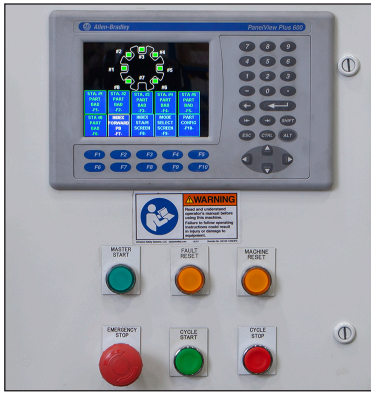
HMI Control Panel
