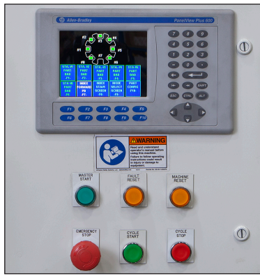
Panel de Control HMI
